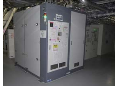
External view of a heater abatement system
