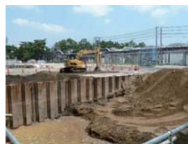
A scene from the excavation and removal work on the contaminated soil
