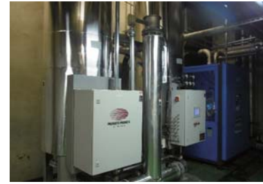
Heating drying machines
