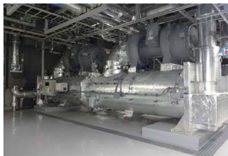
Exterior of the cooling machine
