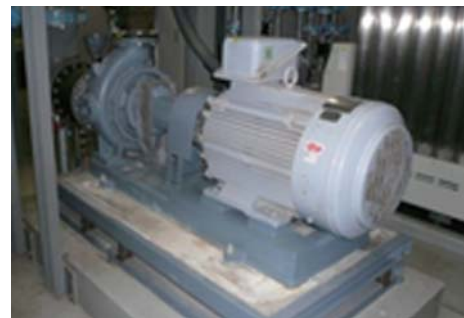
Exterior of the cooling water pumps
