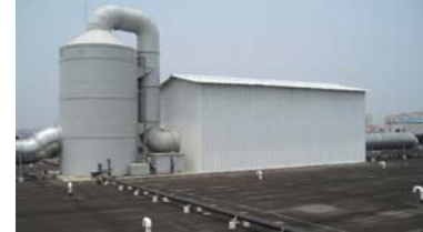
VOC abatement equipment
