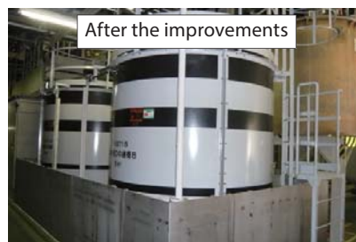
Visible water tanks
