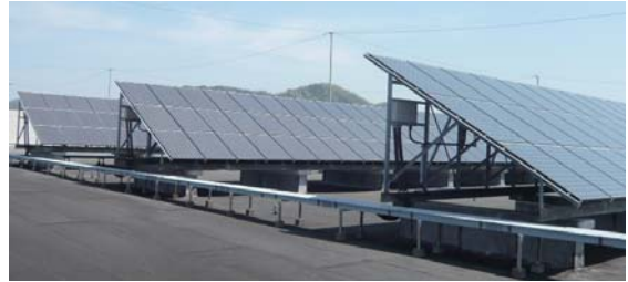
Solar power generating panels at our Tottori Plant
