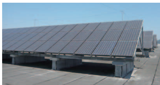
Solar power generating panels at our Tottori Plant
