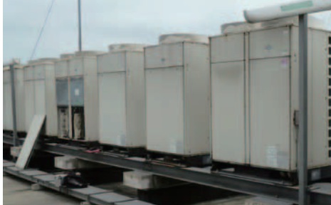
External unit of an air conditioner using fluorocarbons
