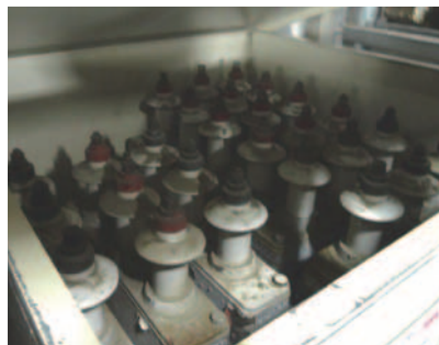
PCB waste (large condensers in packaging)
