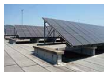
Solar power generating panels at our Tottori Plant
