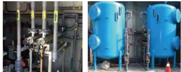
Equipment for recovery and reuse of wastewater from the production process
