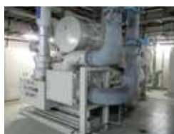
Building F, second floor refrigeration unit
