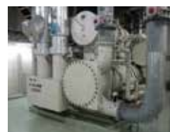
Building F, fifth floor refrigeration unit
