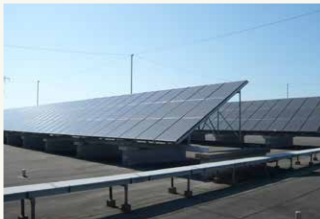
Solar power generating panels
