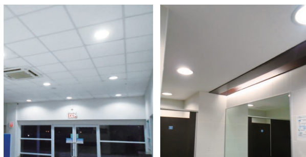
Example of Energy-Saving Improvements: Shift to LED Lighting
