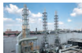
VOC Scrubbing System for D2 Building
